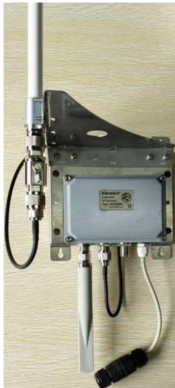
Figure 3-6 4G antenna installed
