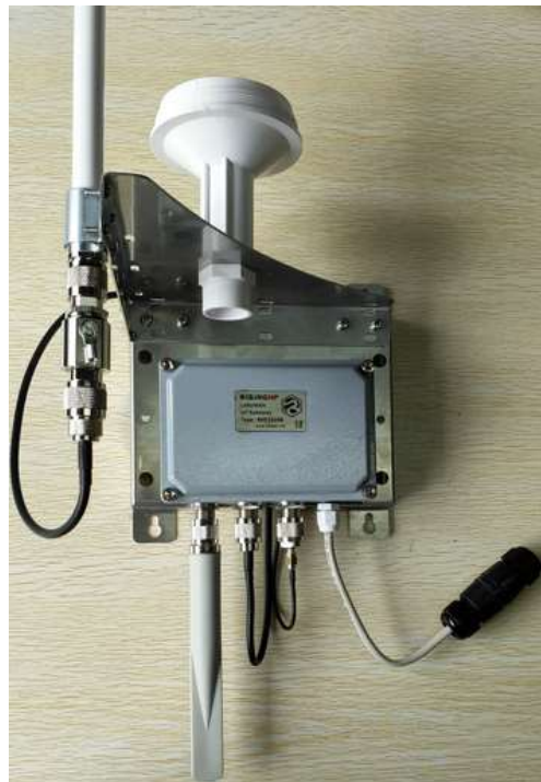
(2) GPS installed with cable connected
