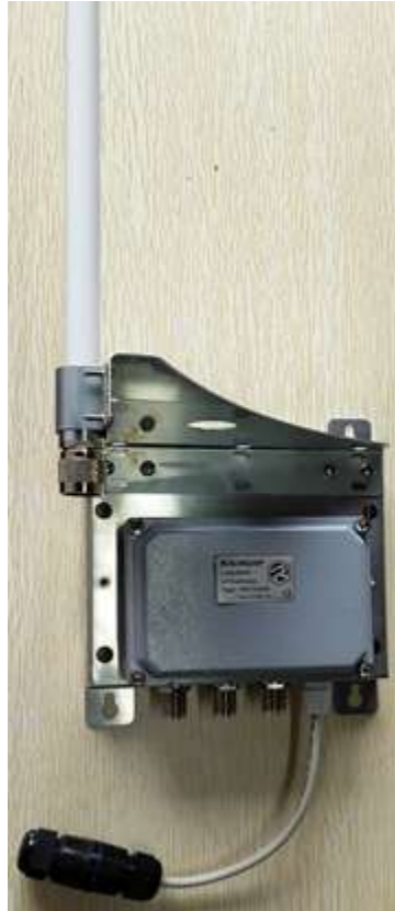
(2) LoRaWAN antenna fixed
